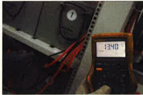
Figure 3. Voltage Measurement on Battery
