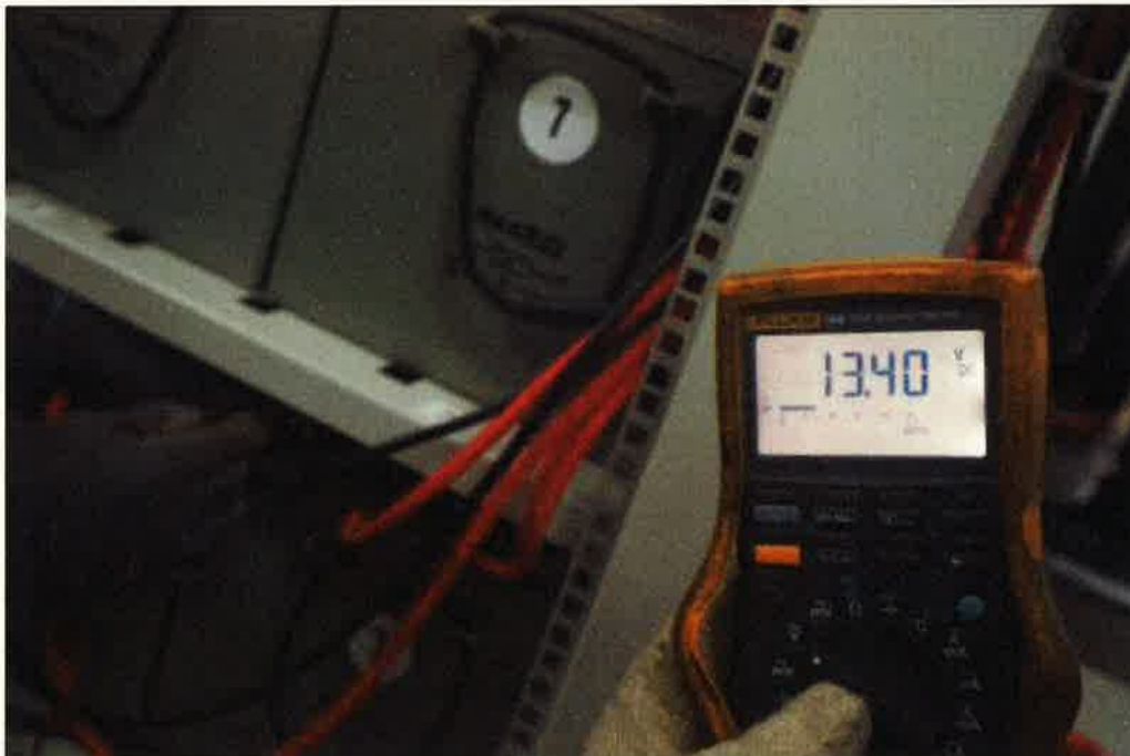
Figure 3. Measurement on Per Block Battery
