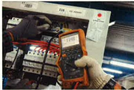
Figure 2. Voltage Measurement of Rectifier Output for Battery and Load
