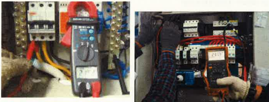
Figure 1. The measurement of Phase Voltage
