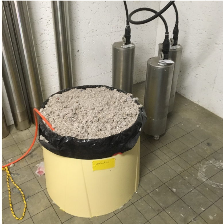
Figure 3 Picture of installed seismometers, before insulation
